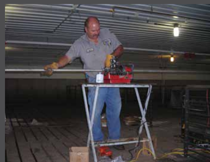
Levi Ringquist (top) and Brian Rons (bottom) use their piping skills to bring an empty hog barn back to life.
